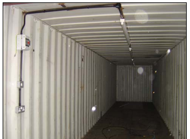
40' Standard - Electrics & Lighting
